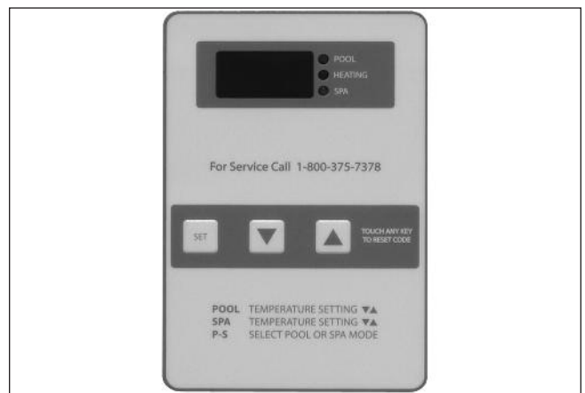
Fig. 5: Digital Water Temperature Control
